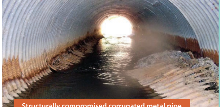
Structurally compromised corrugated metal pipe
